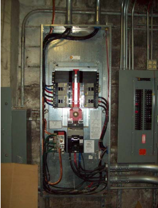
Fig13. Existing 400A, 208V, 3-phase MDP in Excellent Condition
