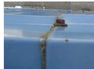
Fig.4 Corroded metal fasteners
