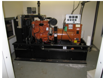
Fig.11 Backup generator for First Bank
