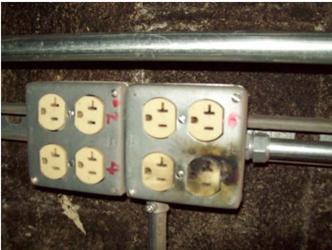
Fig18. Receptacles in Poor Condition
