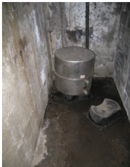
Fig.9 Foundation water seeps
