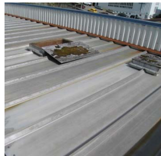
Fig.3 Deteriorated roof hatches
