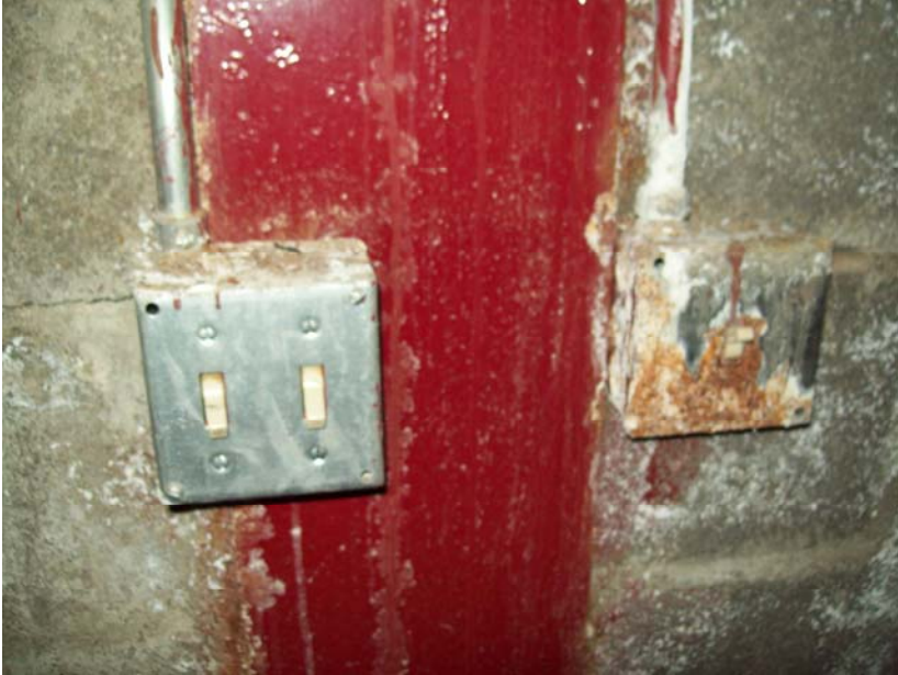
Fig.19: Light Switches in Poor Condition
