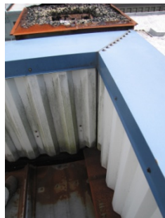
Fig.2 Corrosion of roof metal caused by fire station stack gases
